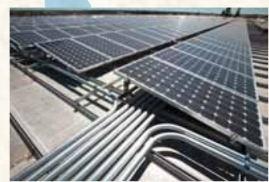
8. Rocklin, CA Roof boasts a 1.2 Megawatt solar array, offsetting over 60% of electricity needed to run the building's refrigeration unit.
